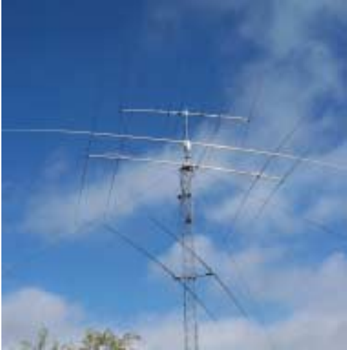
A single tower at AE6Y supports the three, Force 12 antennas, and a fixed-position, 2 element SteppIR.
