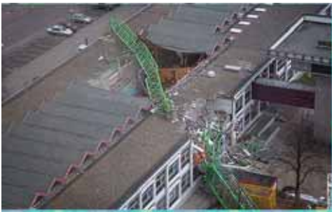
Tower crane toppled by winds in Europe. (all photos, Charles, M0OXO)
