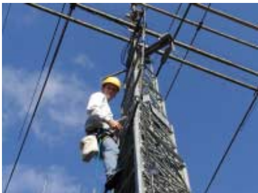
Dean, N6DE, on N6TV's tower fixing the coax to the 10 meter antenna. Now, maybe there'll be some SS activity on 10.
