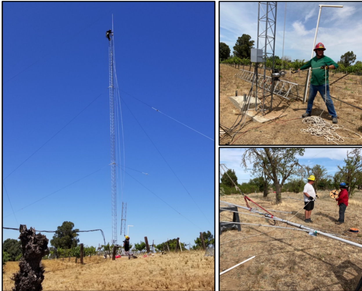
Figure 10. Left, hoisting a tower section. Lower guys are already tensioned. Upper right, the winch operator (KK6PXT) has a lot of responsibility. Lower right, preparing to tram a 10m Yagi.
