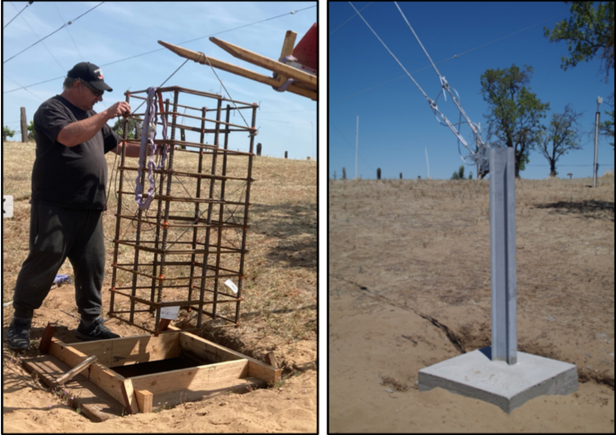
Figure 5. New guy anchors have a substantial rebar cage in the base and use galvanized I-beams that are designed to handle the full load with a large safety factor.
