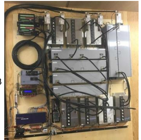
Switching Network at K6MTU
