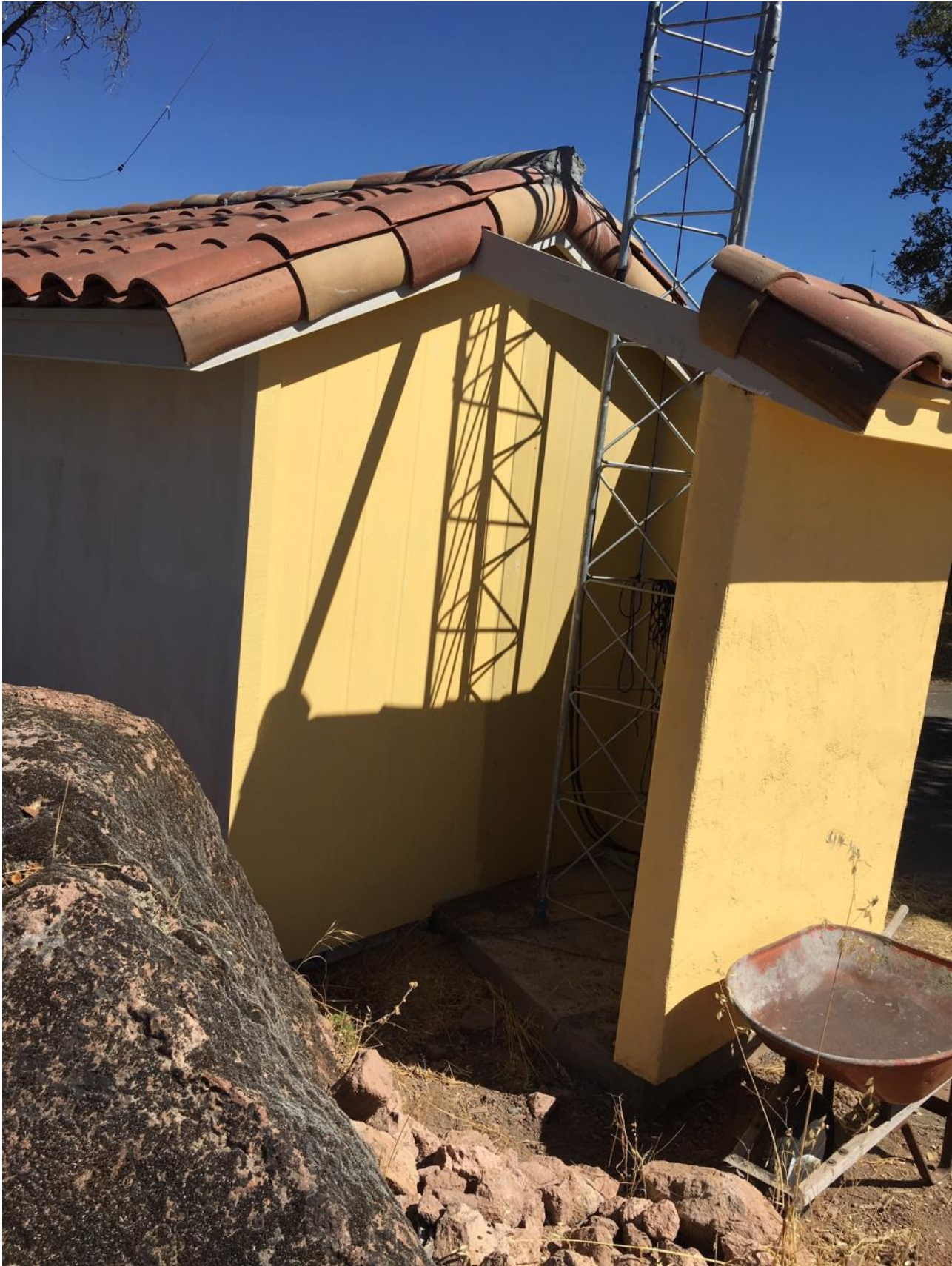
The cut out section of the shed allows full access to the tower.
