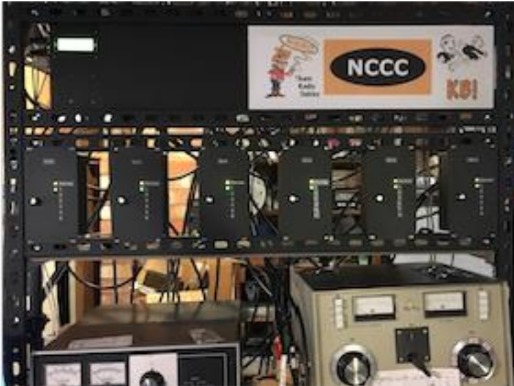
Figure 8. Front of the switching rack.
