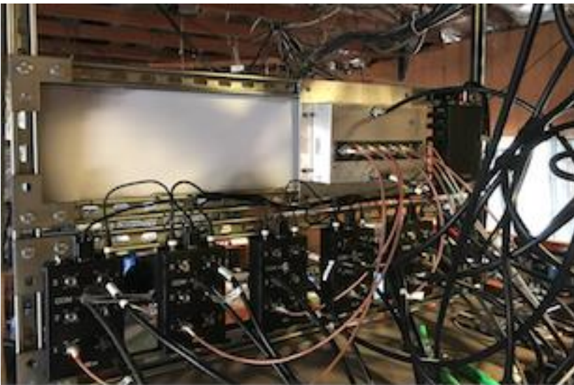
Figure 9. Back of the rack.
