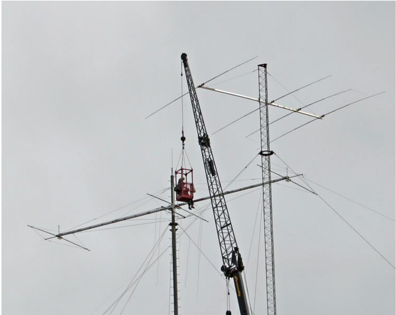
Figure 5 – The “NV’s” sawing off broken elements and cutting trusses. One of the stacked 4 element 20M beams in the background.
