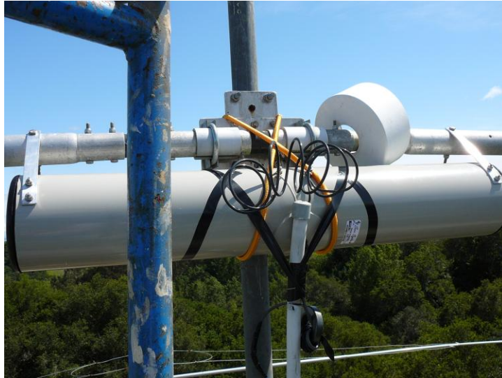
The Eight Pak installed on Sigma 180 S
